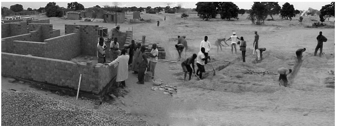
PHOTO 1 Self-help building in a zone of auto-construção on the periphery of Luanda
