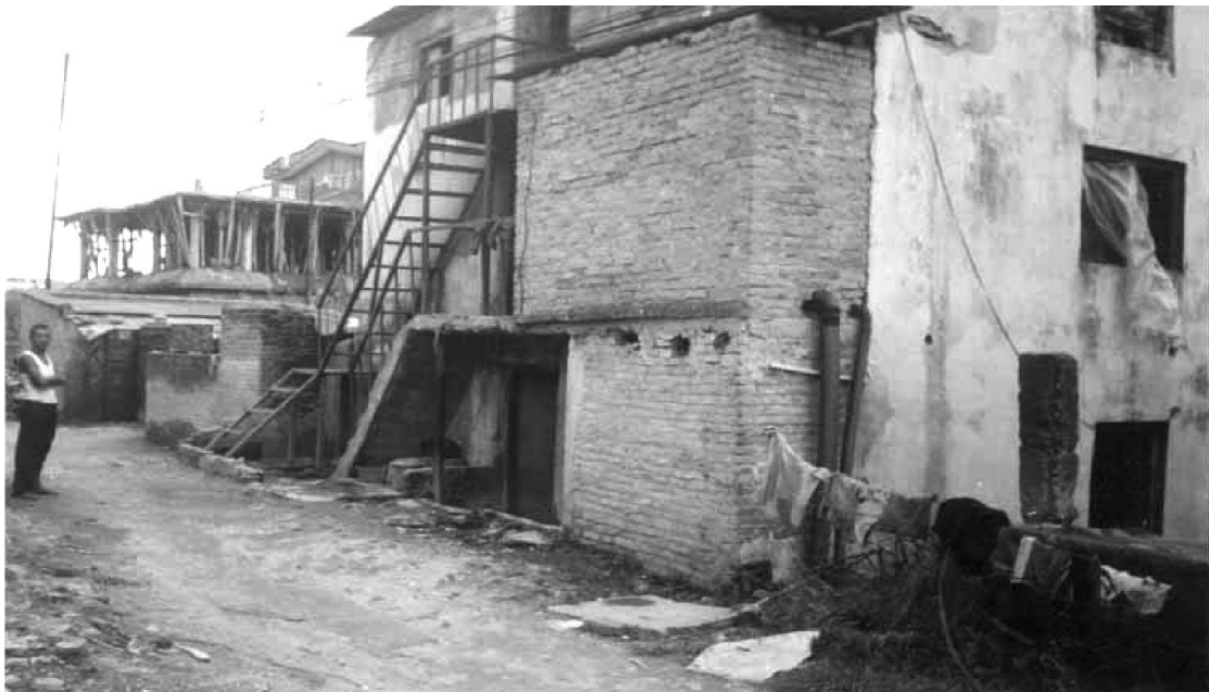
Photo 1: Illegally encroaching portion of a building still standing one year after the initial demolition operation
