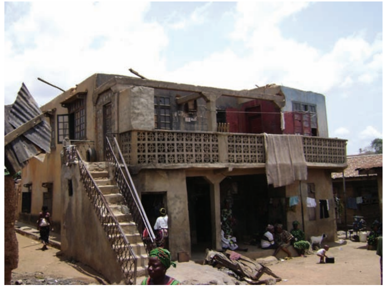
PHOTO 1 Wind-damaged building in the core area of the city, with its roof totally blown off
