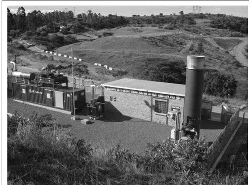
PHOTO 1 Landfill gas-to-electricity installation © Durban Cleansing and Solid Waste Department, eThekweni Municipality
