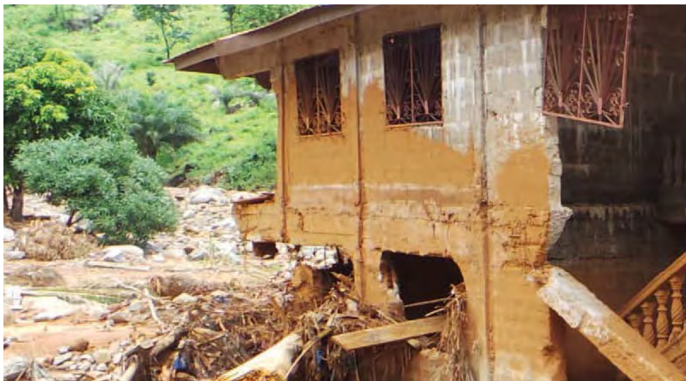
Landslide and Building Collapse. Photo Credit: World Bank Assessment on Landslides and Floods in the Western Area, 2017.
