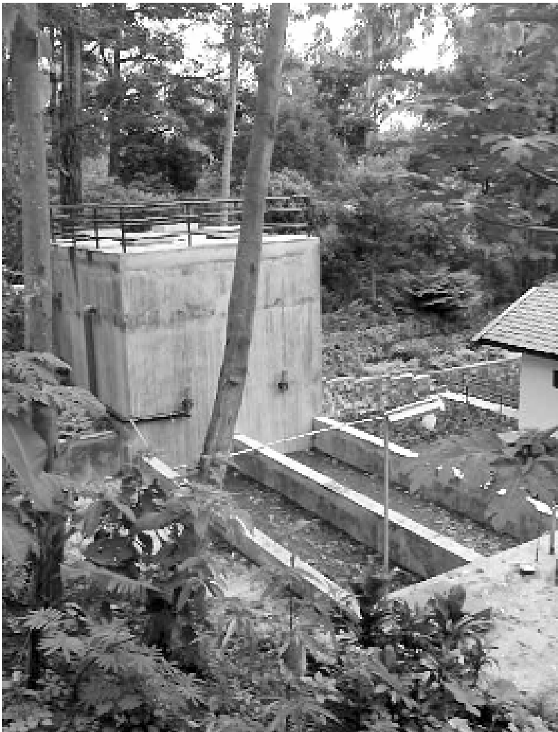
Photo 6: Wastewater treatment system at the kelurahan level in Malang, Indonesia
