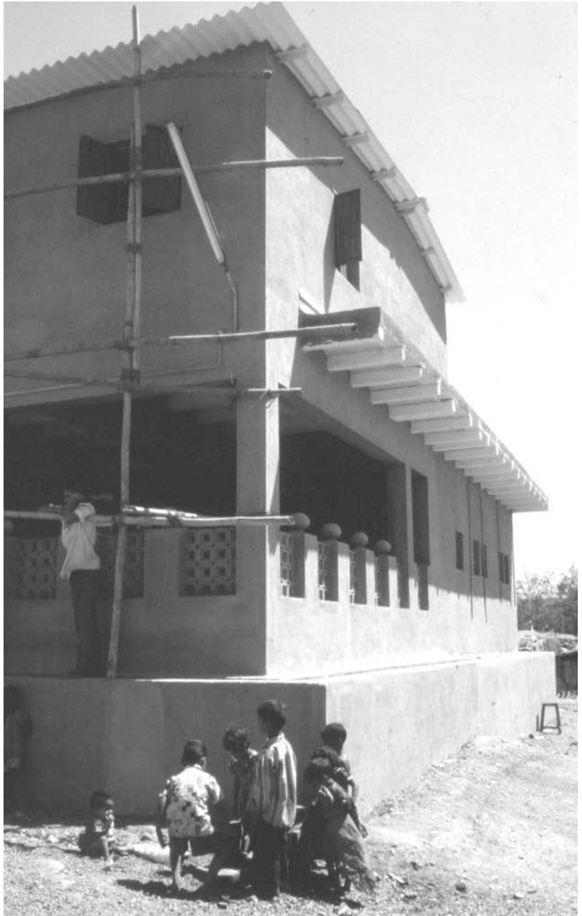
Photo 2: The community-designed Chikhalwadi toilet block in Mumbai under construction. Credit: Homeless International
